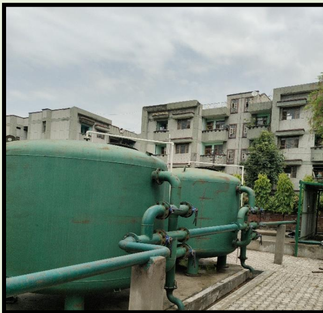
Water Treatment System
