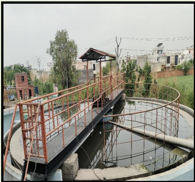
Water Recycling Unit
