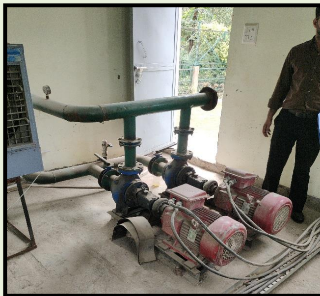
Bore Well Recharge system
