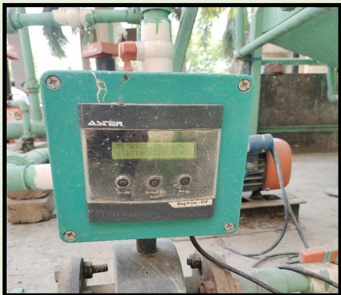
STP/ETP Outlet Reading
